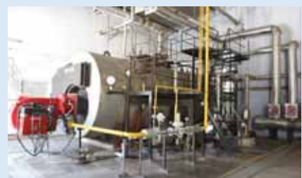
Boilers using Natural Gas at Indrad Facility
