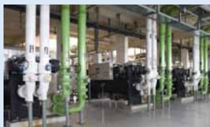
Energy Efficient Equipment at Dahej Facility
