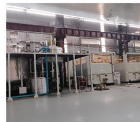
VPI Plant with Oven
