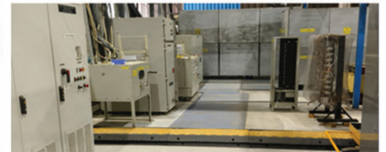
Converter Set up for System Test
