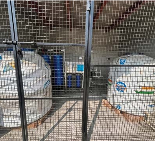
Figure 3: Water Purifier and Water Tanks
