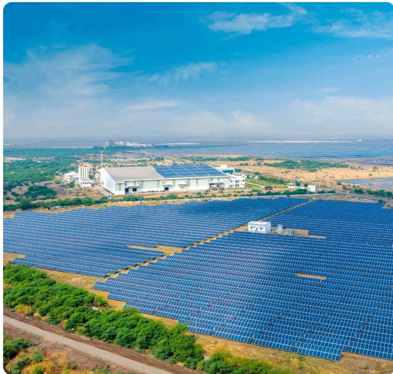
Solar Power Plant, Dahej CZ
