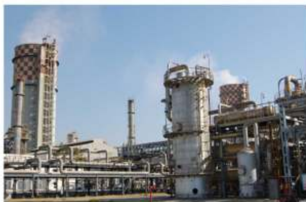
VIJAIPUR I & II PLANT
