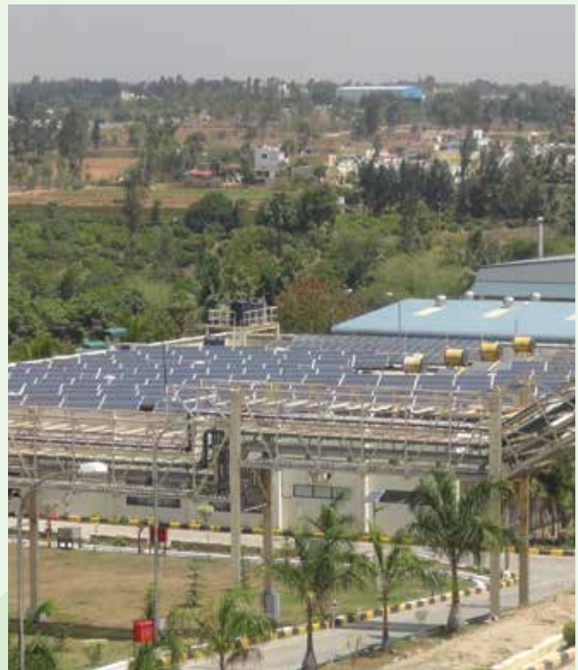
Rooftop Solar at the Sayakha Plant
