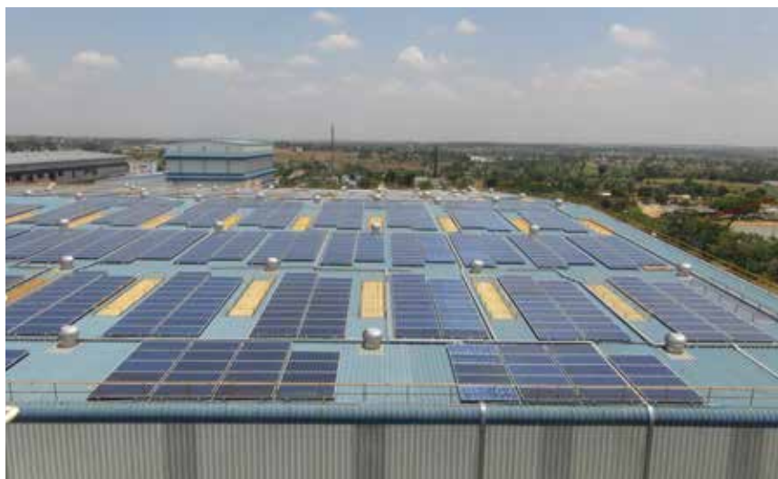
Rooftop Solar at the Hosur Plant
