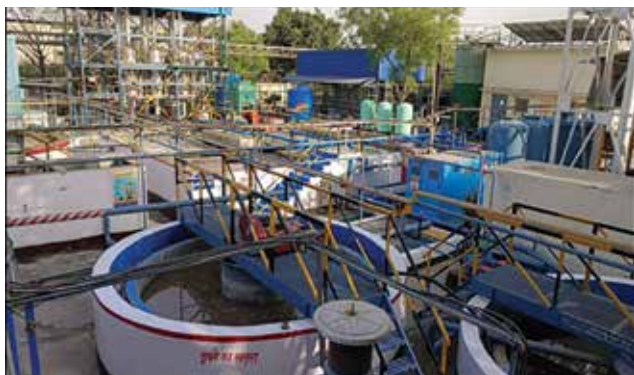
Effluent Treatment Plant at Jainpur Plant
