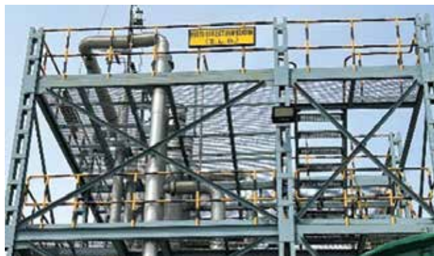
Multiple Effect Evaporator (MEE) at Goindwal Sahib Plant
