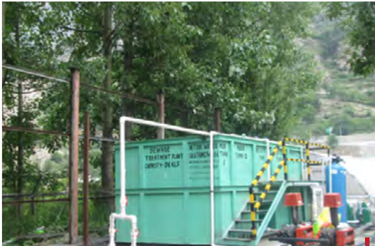
Sewage Treatment Plant at Sholtu
