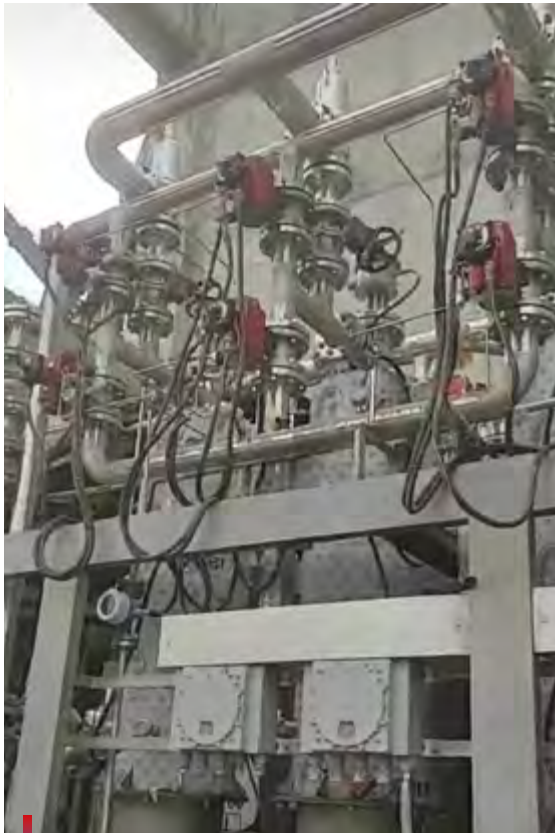
Green Hydrogen Plant, Vijayanagar
