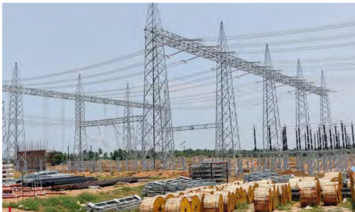
Pooling Station, Dharapuram
