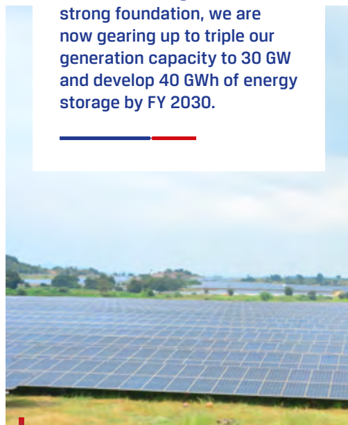
Solar Plant, Vijayanagar
