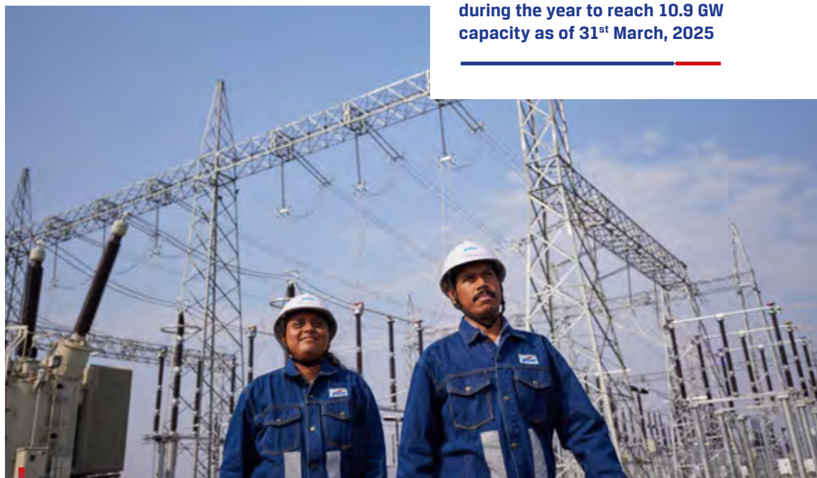
Solar Power Plant, Vijayanagar
