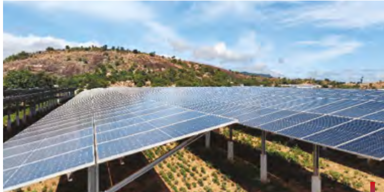
JSW Neo Energy
