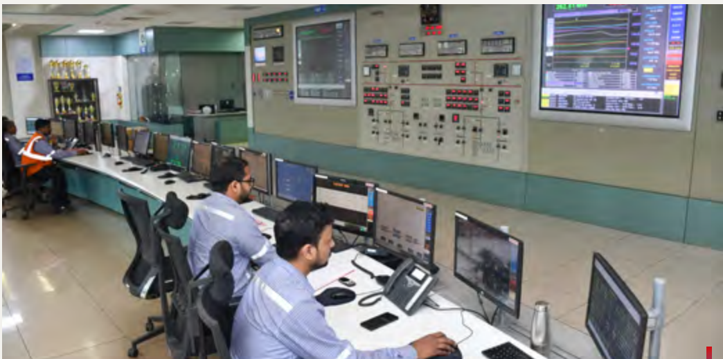
Thermal Power Plant, Ratnagiri
