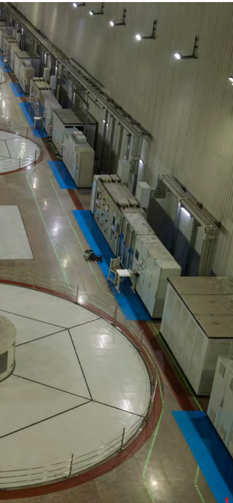
Turbine Floor, Baspa-II Power House
