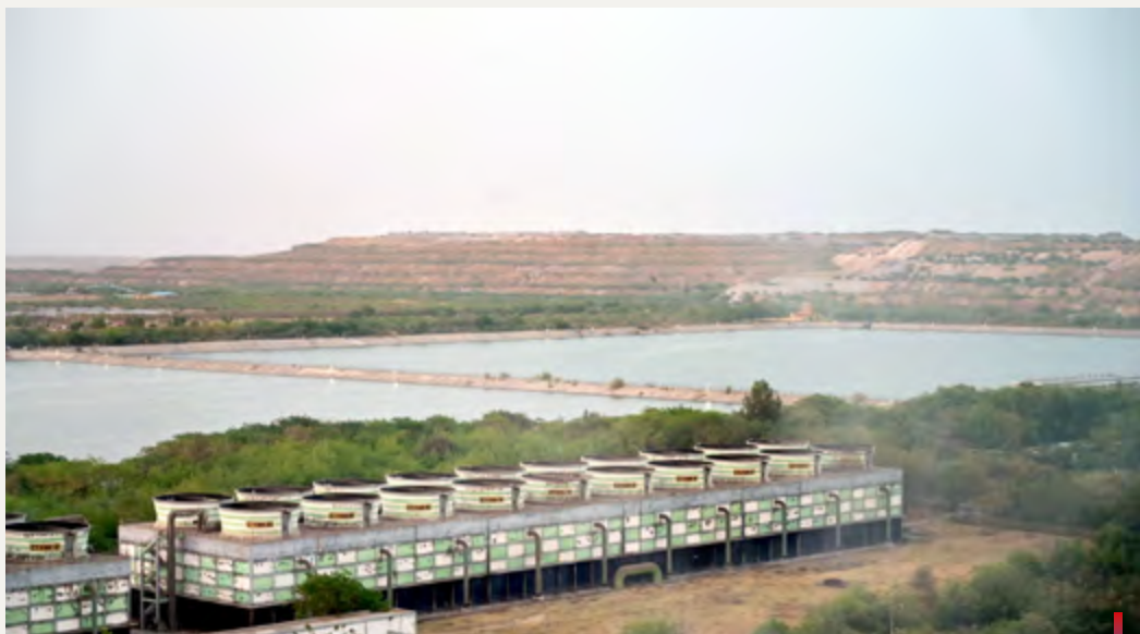
Barmer Power Plant
