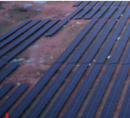
Solar Plant, Vijayanagar
