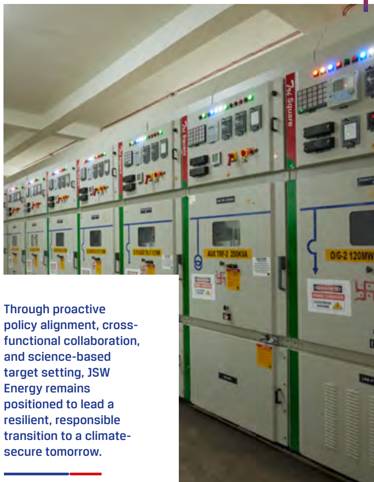
Electrical Panel Room
