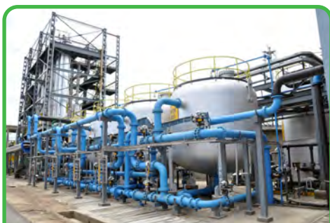
Complete Zero Liquid Discharge
