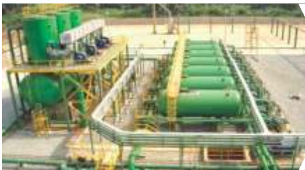
Pretreatment at OKPAI Power Plant, Nigeria
