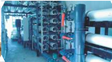
Desalination Plant for Al Ghubrah Power, Oman
