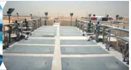
Membrane Bio-reactor Plant at Industrial Area, UAE
