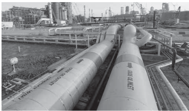
Crude Oil Pipeline at Paradip Refinery
