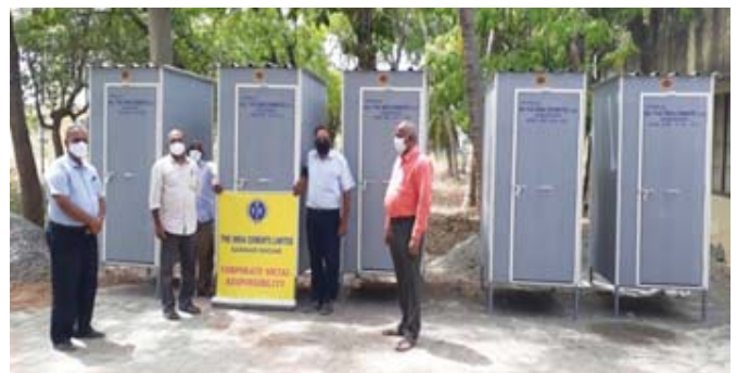
Mobile sanitation facilities for migrant workers
