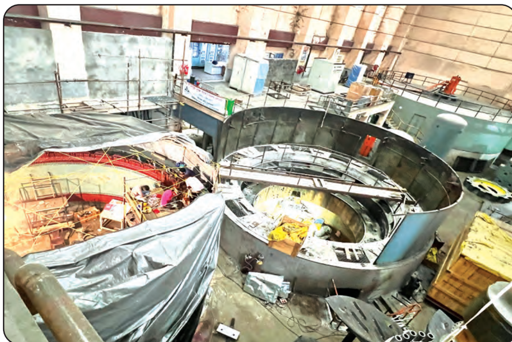
Damodar Valley Corporation for Renovation, Modernisation & Up-gradation of Panchet Hydel Unit-1 (40 MW), Panchet, Jharkhand
