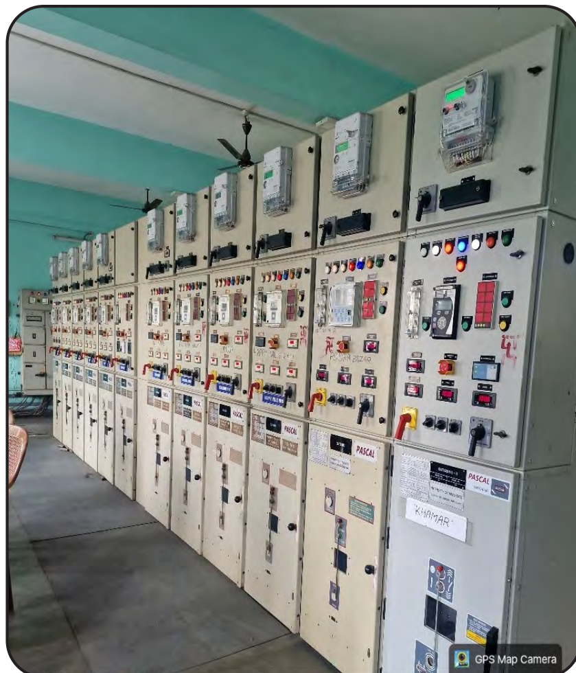
Safety Enhancing System Improvement Scheme (SESIS), for Electricity Distribution Across West Bengal.
