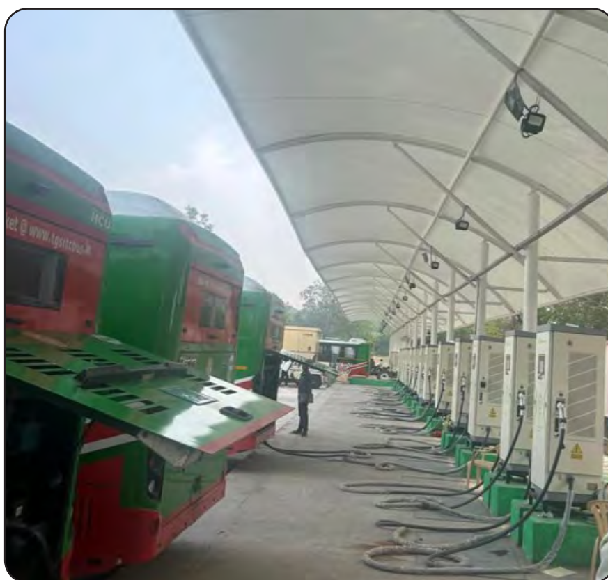
Charging Stations in Bus Depots, Hyderabad, Telangana
