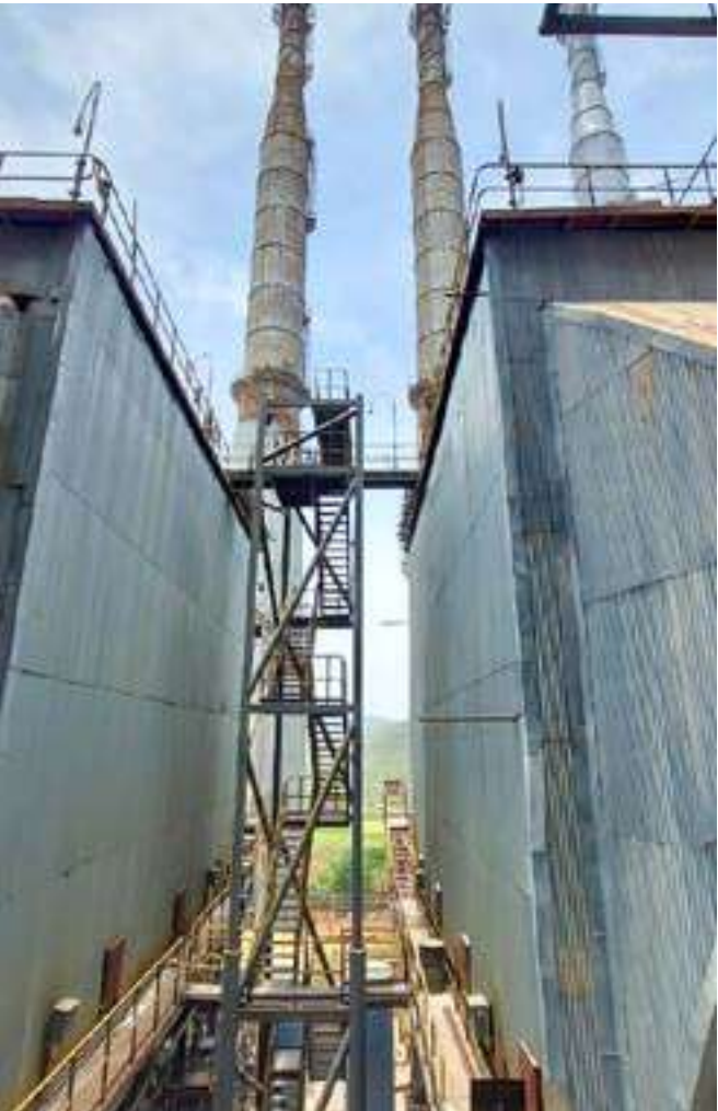
Calciner stack and ESP at Utkal Alumina
