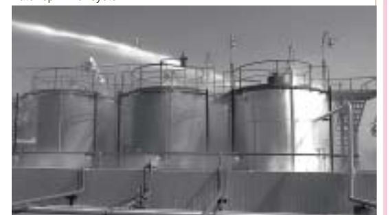
water sprinkler system
