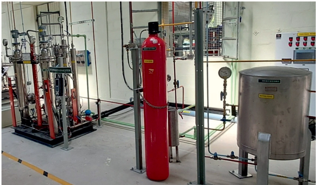
HYDROGEN COMPRESSION & STORAGE
