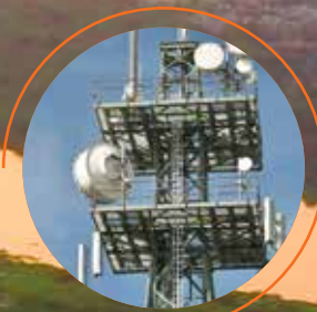
5G Telecom Towers
