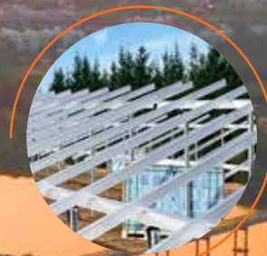
Solar Mounting Structures
