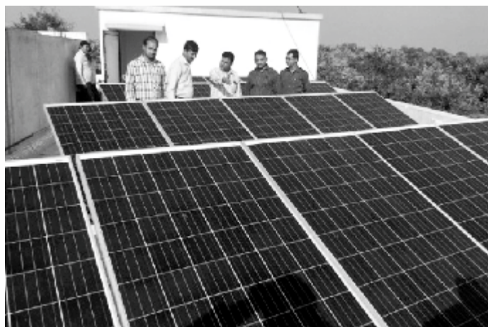
Solar panel at CNG station
