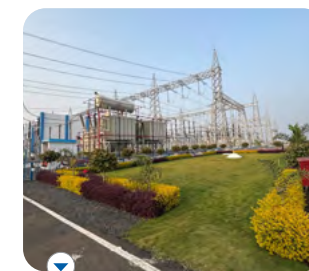
Transmission System in Rajgarh (BOOT)
