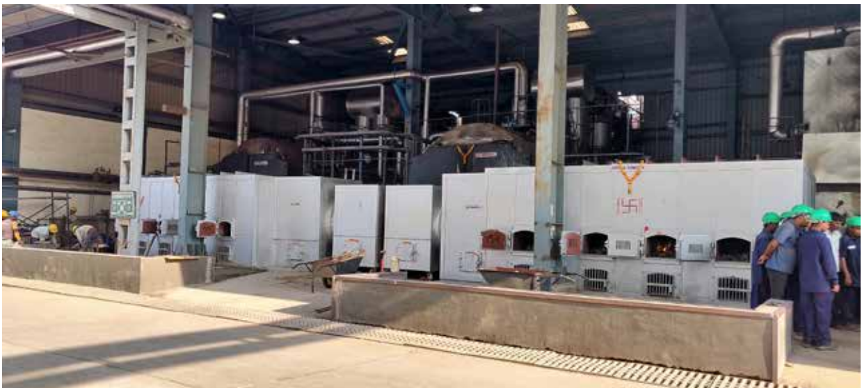
Briquette boiler at Ambernath factory
