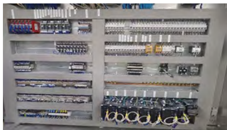
Panel with RCCB & overcurrent protection
