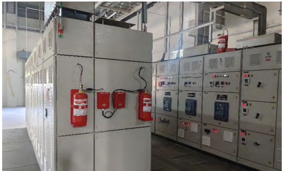
Panel for Fire protection
