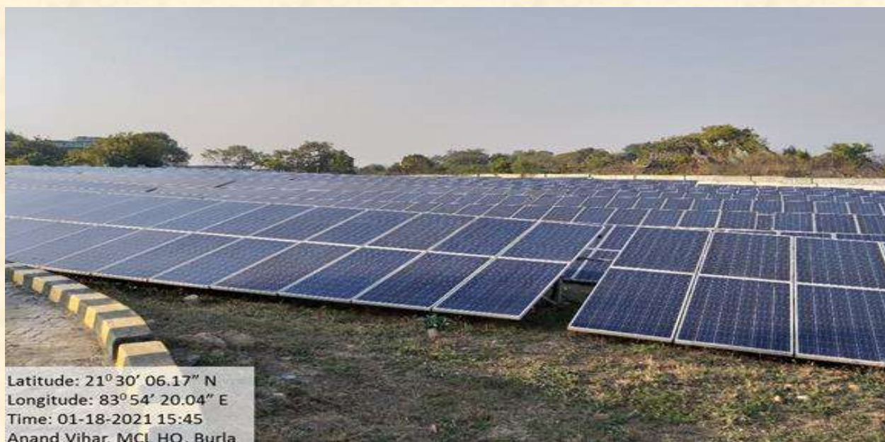
Fig. 49 – Ground mounted solar power plant in MCL
