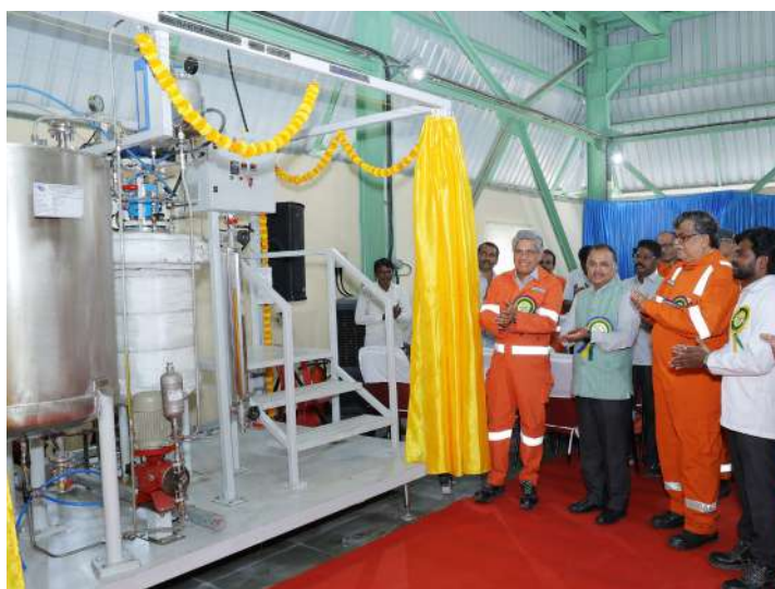
The demo plant which is used to produce Corrosion Inhibitor to mitigate corrosion induced by Ethanol-Blended Petrol was commissioned in December 2024 at CPCL R&D.
