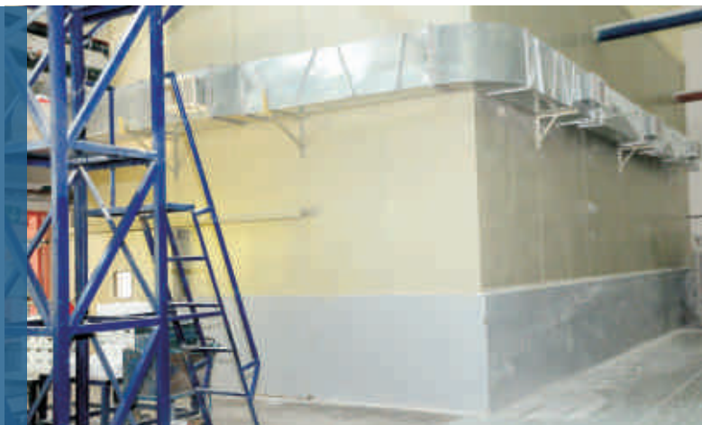
The decentralized exhaust system at the Naganathapura Plant.
