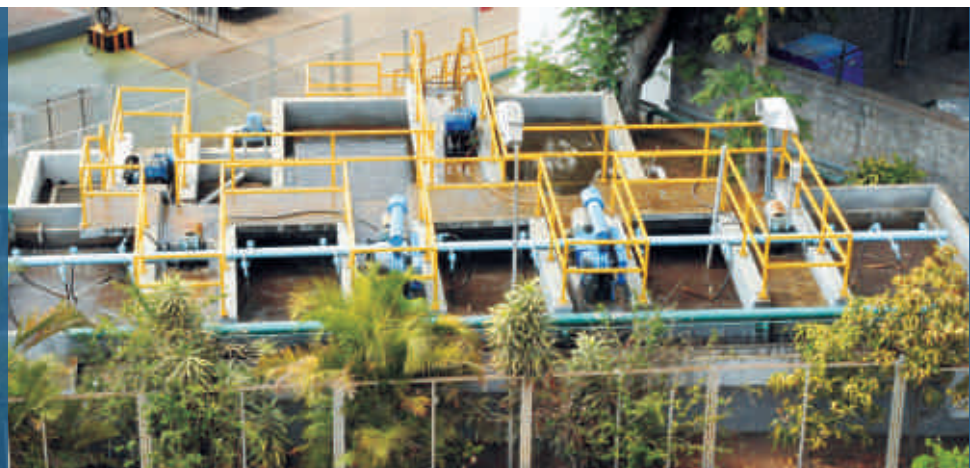
The sewage treatment plant at the Bangalore Plant recycles and reuses domestic waste water.
