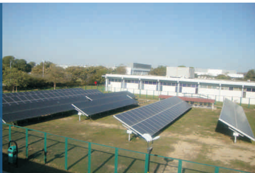
The Jaipur Plant's 40kW solar plant generates around 110 units of electricity a day.
