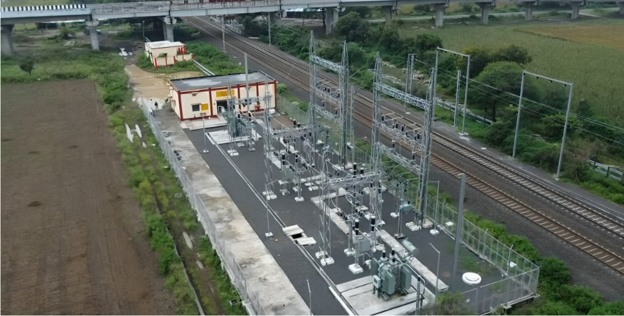
Enabling faster rail connectivity through Sub-Sectioning Posts (SSPs) for the 2x25 kV system on the Mumbai-Delhi route
