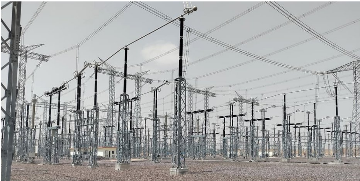
Powering India's future through one of the largest air-insulated substation projects at the 765 kV/400 kV/220 kV PGCIL Substation in Fatehgarh, Rajasthan
