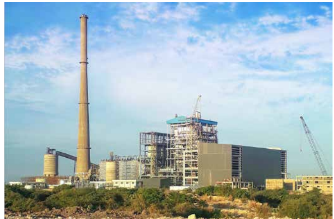
1x125 MW Sendou Thermal Power Project, Senegal
