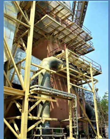
Seawater FGD system for Trombay 1x250 MW
