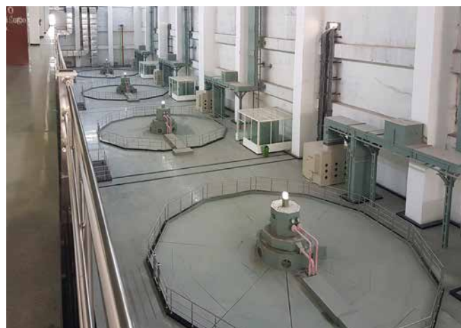
Bay hall of 4X30 MW Pulichintala hydroelectric project in Telangana, commissioned by BHEL
