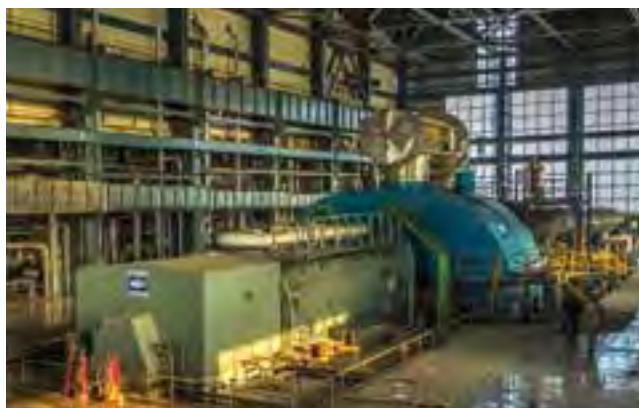
Turbine hall of 700 MW supercritical unit at Bellary STPS, Karnataka
