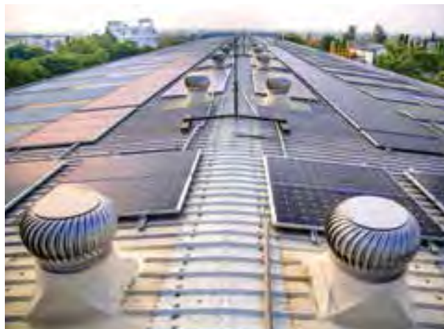
160 kW rooftop Solar PV plant commissioned by BHEL at Hyderabad, Telangana
