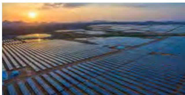
50 MW Solar Power Plant commissioned by BHEL at Kadiri (Ananthapur), Andhra Pradesh
