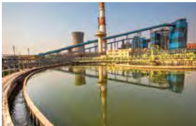
Clariflocculator for Pre-treatment plant commissioned by BHEL at Bellary STPS, Karnataka
