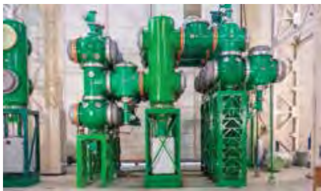
420 kV GIS for NHPC Chamera, Himachal Pradesh, indigenously designed by BHEL
