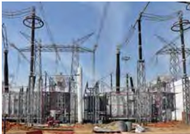
500 MVA 765/400/33 kV auto transformer at 765 kV Greater Noida substation
