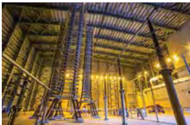
World's first 800 kV pre-engineered Indoor DC hall at NE-Agra HVDC terminal
