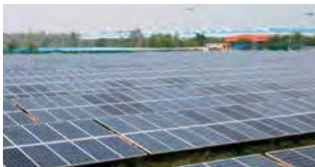
5 MWp captive solar power plant at BHEL Tiruchirappalli, augmenting in-house generation of green power
