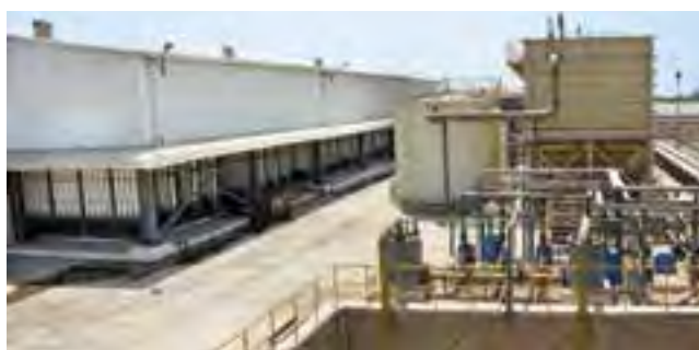
96 MLD Raw Water Treatment plant set up by BHEL at OPaL Dahej Petrochemical complex, Gujarat
