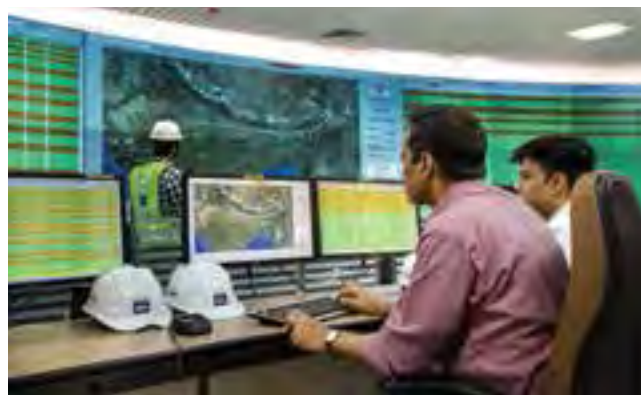
Central control room at Agra converter station of the world's largest ± 800 kV, 6000 MW UHVDC multiterminal North-East Agra transmission link, being executed by BHEL on turnkey basis
