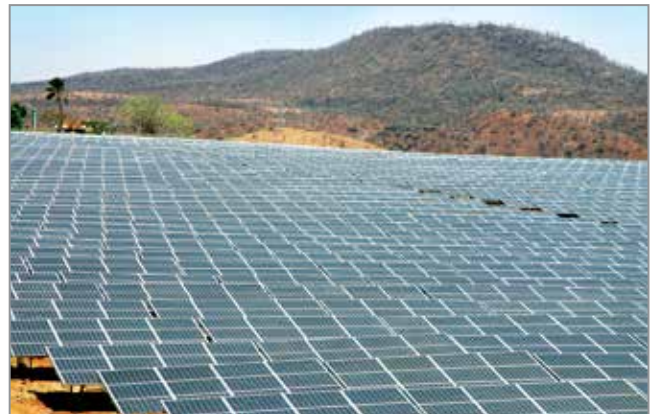
Grid-connected 5 MW Solar PV plant in Karnataka
