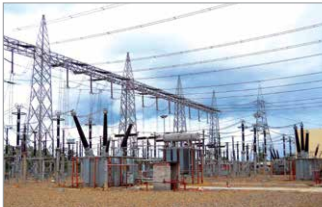
400 kV Substation at Gas-based Power Plant, OTPC-Palatana
